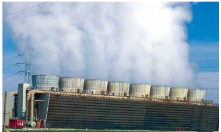
Figure 1: Cooling Tower Plume
